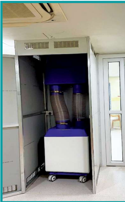
A State-of-The-Art BMT Unit In one of The Foundations In Bengaluru
