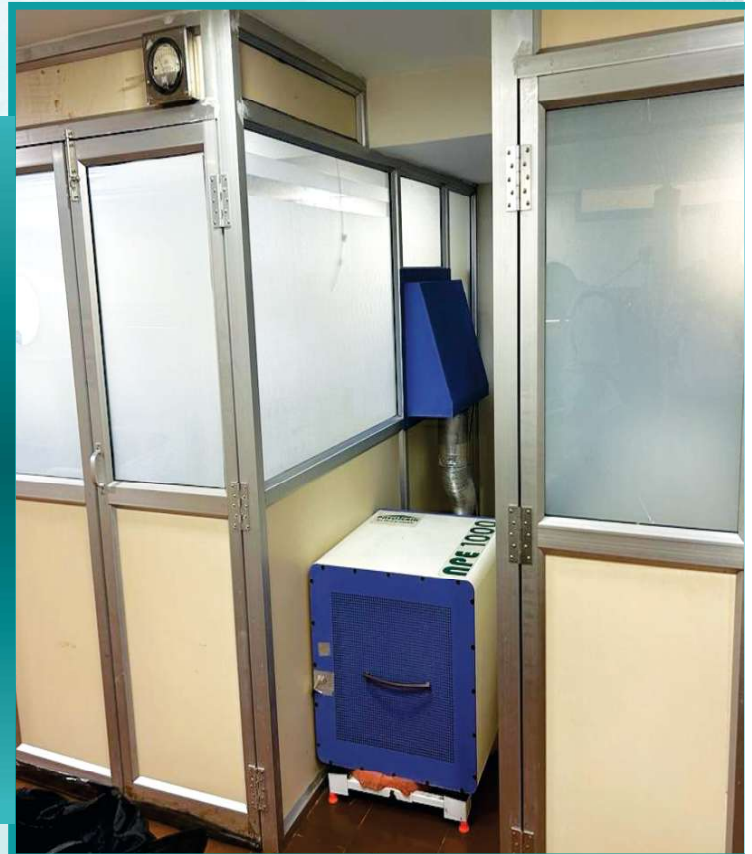
Negative Pressure Enclosure at a Multi Speciality Hospital In Chennai
